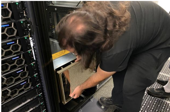
Thomas Olson Helping Install the CEOAS DGX-H100.
